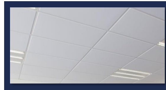
Attachments to floors, ceilings, internal walls and internal linings of external walls
