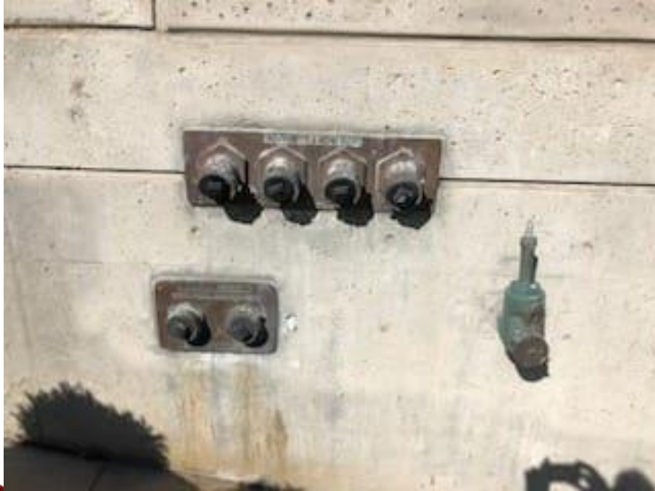
Medium rise dry hydrants in San Francisco
