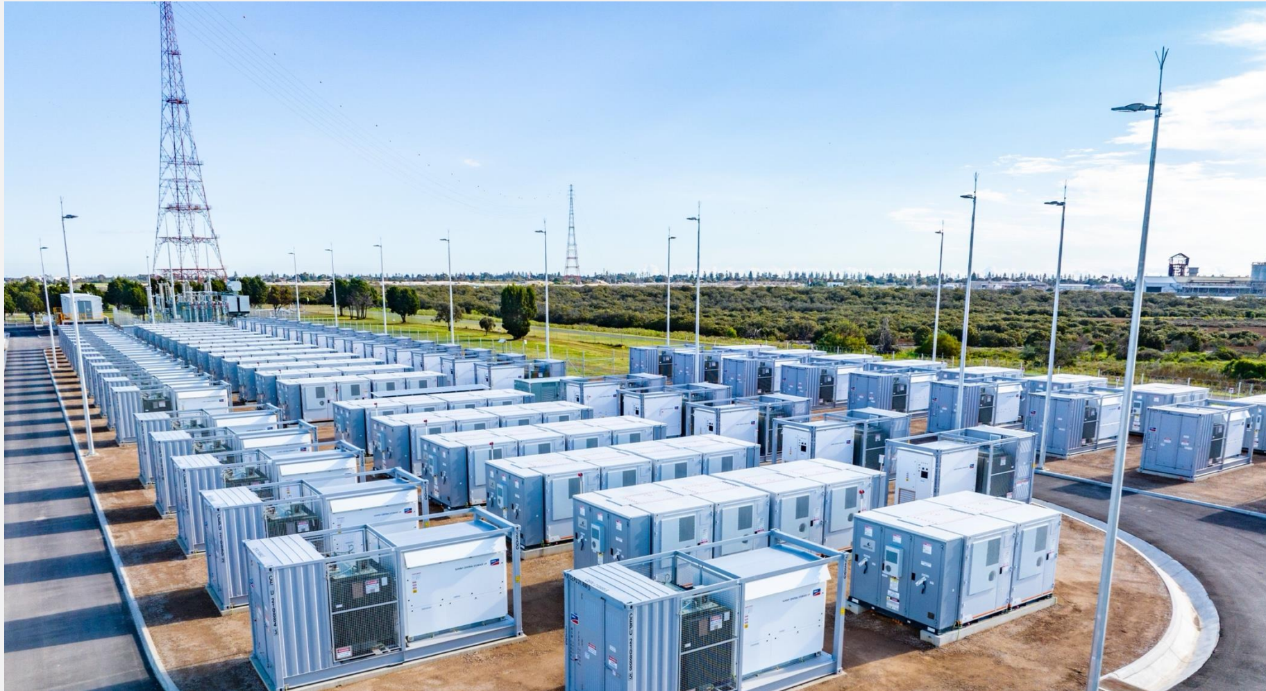
Millions of battery cells comprising a large-scale BESS
