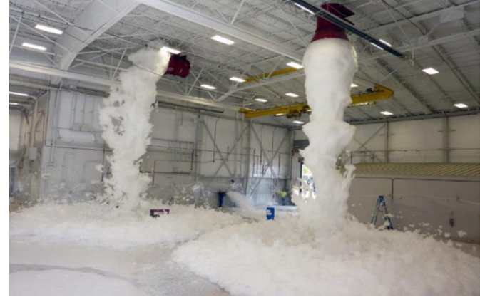
High-Expansion Foam Deluge System Discharge [image courtesy Global Aerospace (2026)]
