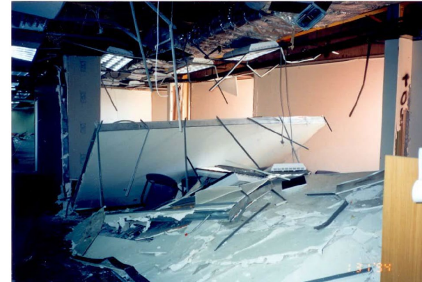
3. Ceilings pulling walls down
