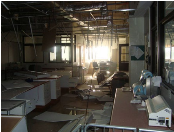
4. Ceiling connections failing
