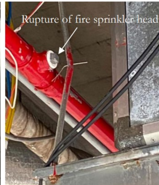
Figure 7. Rupture of sprinkler head
