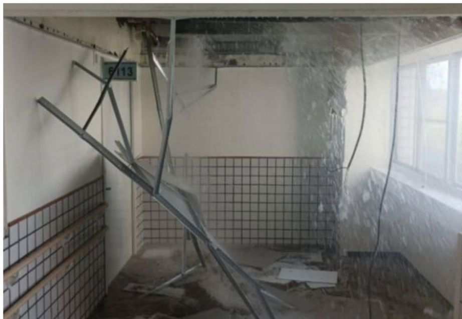
Figure 4. Failure to fire sprinkler heads
