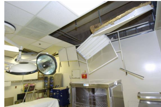
6. Dislodged supported services
