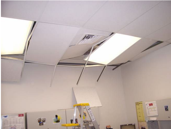
1. Ceilings torn from walls
