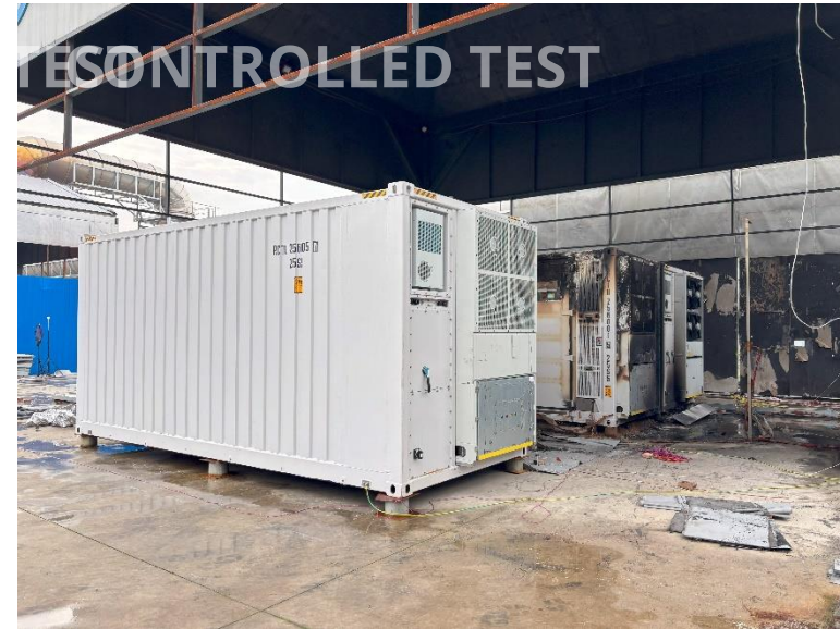
Back side of Container 4 and view of chillers of Container 4 (left), Container 5 (middle), and Container 6 (right)
